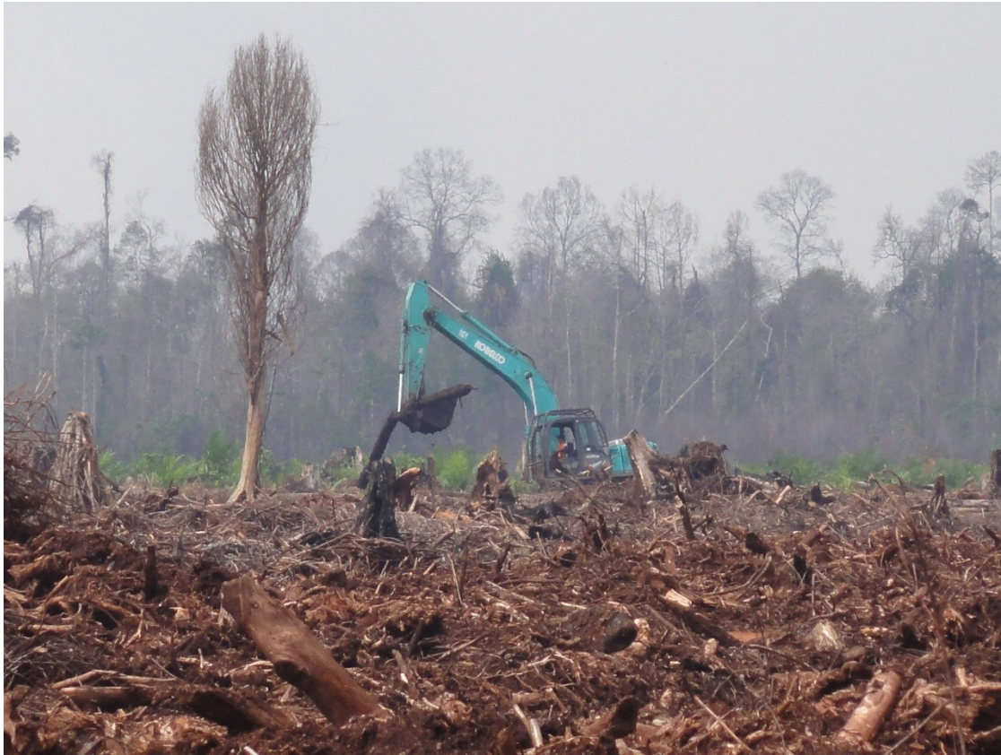
Excavator used to clear land in the concession of PT. SRL Block IV Rupert Island. The coordinate is at N1°48'23.74" E101°37'50.18". Photograph taken on 17 July 2014 by WWF-Indonesia Riau Program.
